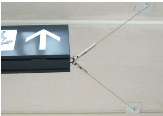
Vibration stopper in station
